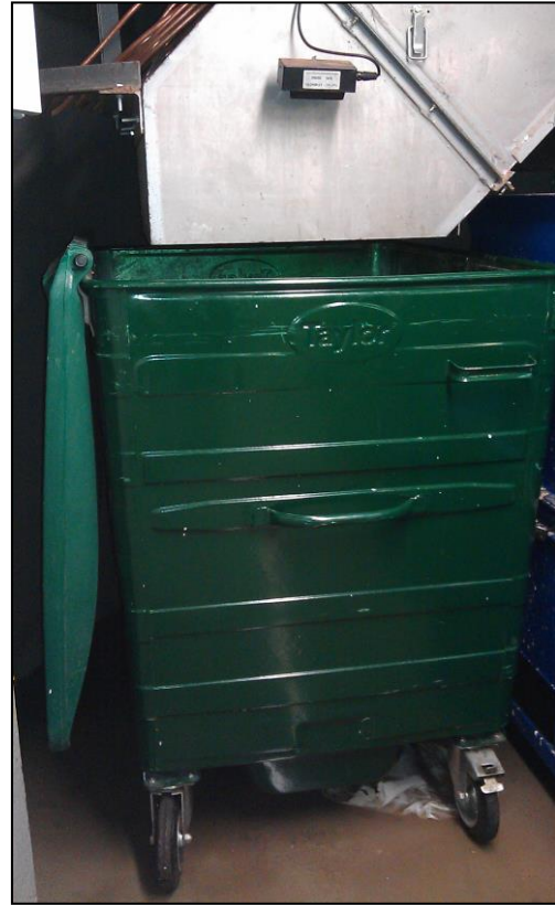
Chute-fed dry recycling container
